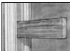
Two ways of attaching second story porch joists to Old South columns.
